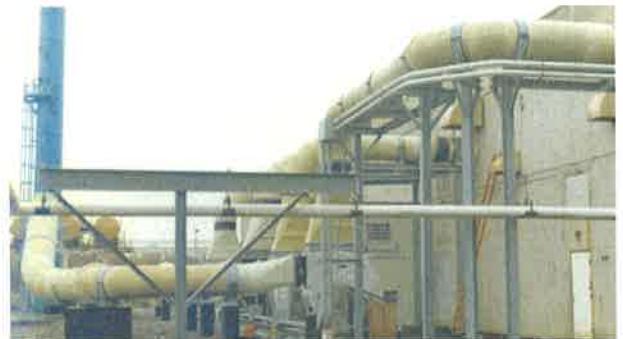
Hot Air Exhaust 5' dia. Hot air exhaust duct to FRP stacks
