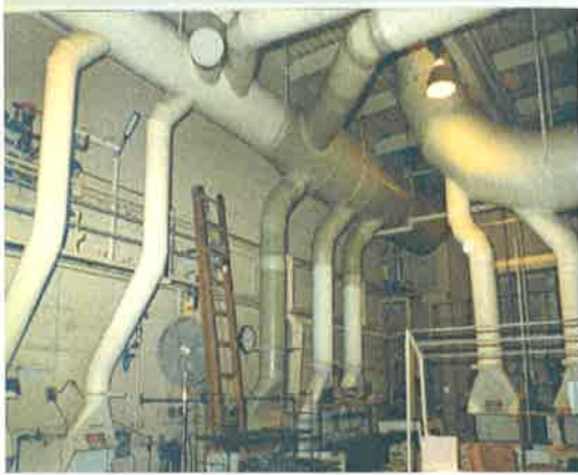
Exhaust System for Plating Operation Complete System with plenums, 8", 10" & 12" risers and 16" & 24" exhaust main.
